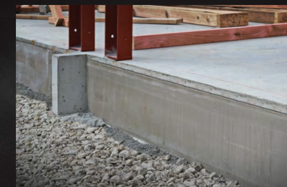
3 Boxing is removed, revealing a truly integrated, aesthetically finished thermal barrier. Once wall framing and cladding is fixed in place, for optimum service life and insulation, two coats of acrylic paint should be maintained to all exposed surfaces.
