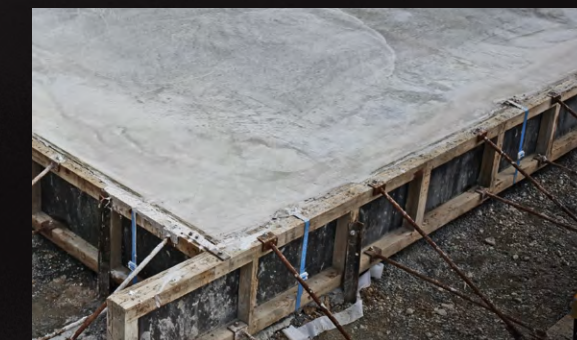
2 RibRaft® RaftMix® concrete is poured covering the angled top edge of the HotEdge® anchoring it into the slab.
